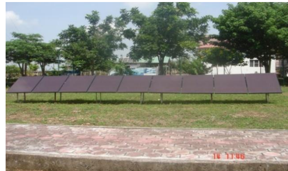
Fig 6: Thin-Film PV panels at RGPV, Bhopal
