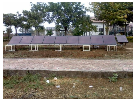
Fig 7: Thin-Film PV panels at RGPV, Bhopal after the installation of GC-CPCS
