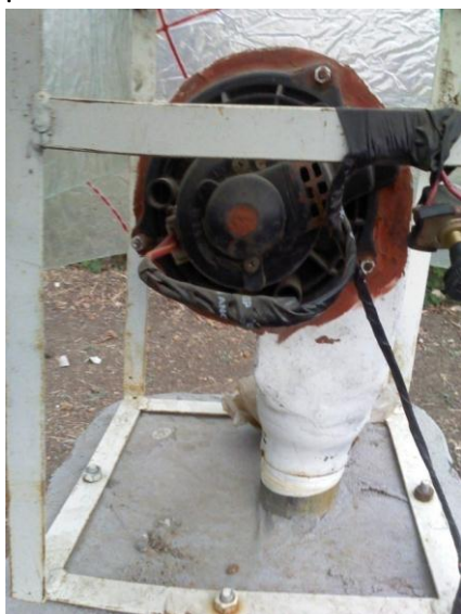
Fig 13: Blower used in the experimental set up
