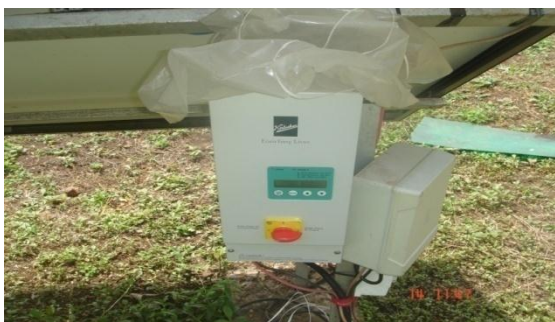
Fig 17: Solar Power Conditioning Unit (SPCU)
