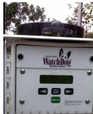
Fig 16: Pyranometer installed in Weather Monitoring Station
