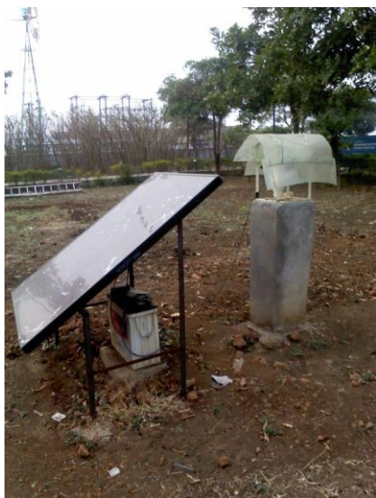
Fig 14: Solar PV panel along with battery and charge controller, dedicated to supply power to the blower
