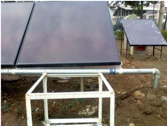
Fig 8: Arrangement of pipe line and support frames of GC-CPCS
